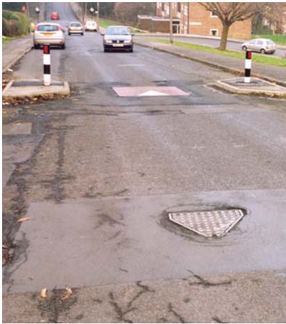
Poorly reinstated traffic calming. Keith Sharples Photography.
