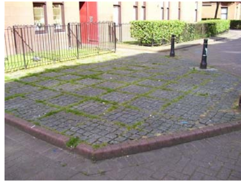
Unightly finish due to spalling and / or weed growth.
