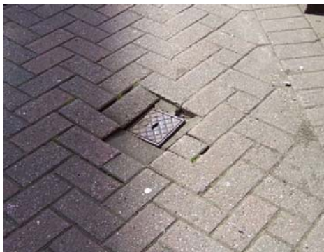
Settlement of blocks surrounding ironwork, leaving the ironwork sitting proud of the carriageway.
