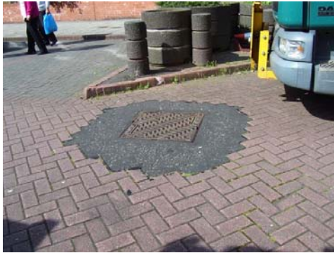
Reinstatements using alternative material i.e. asphalt, concrete rather than blocks.
